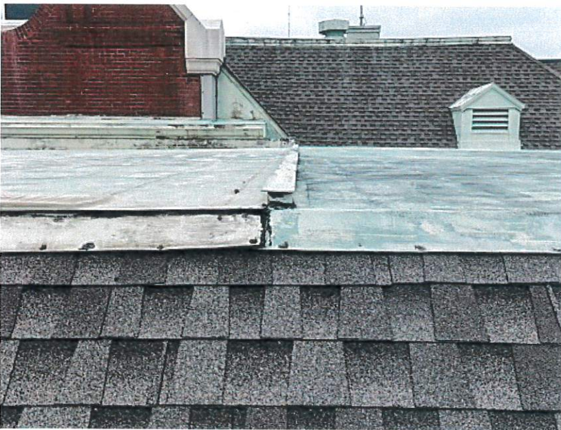
Edge Metal to be repaired
