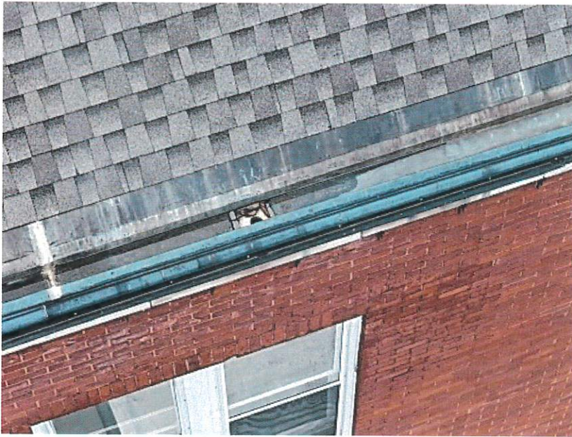
Gutter Drain to be repaired
